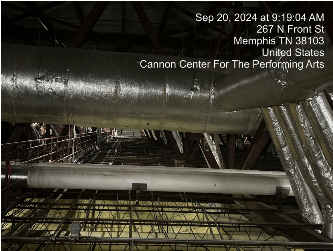
Image 2: Water Lines Above Steel
