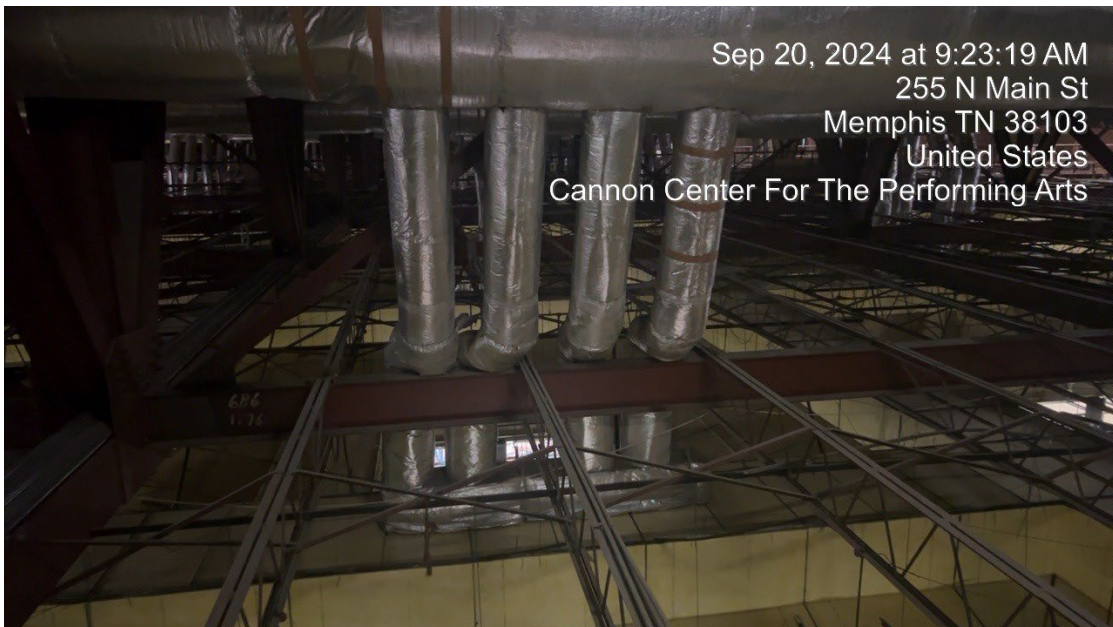
Image 1: HVAC Rubbing on Steel
